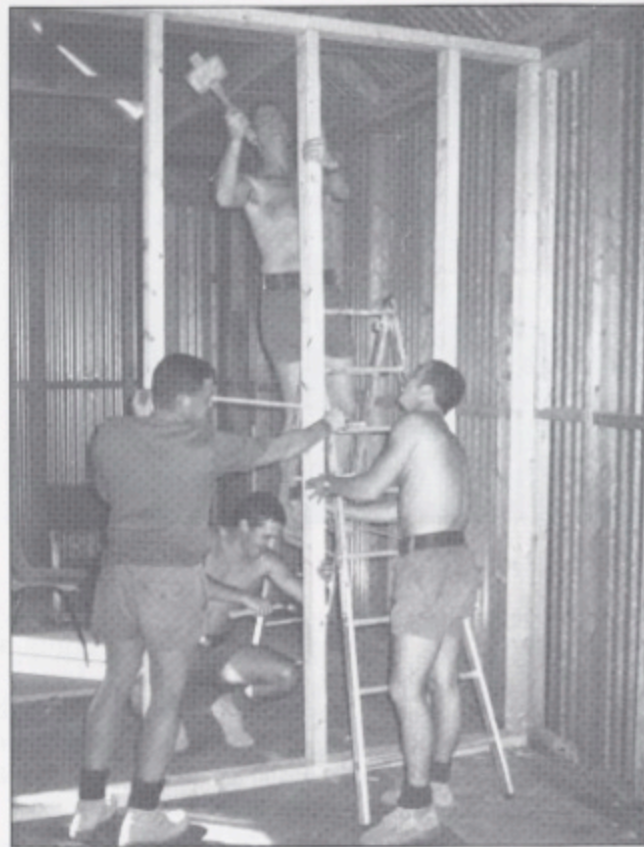
Cpl Blundell, LCpl Doherty and Sappers Naylord and Bowden erecting timber partitions to be later clad with plasterboard prior to decoration.
