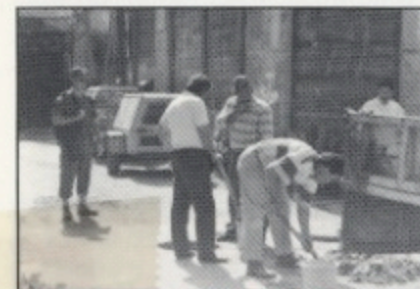
The escort, Bdr Boland, observes some civilians conducting repairs of the sewage system in the Buffer Zone.
