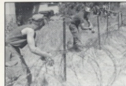
Bdr Sutton and Bdr MacCarthy repair the barbed wire at C84, OP Cockburn near Ledra Palace Hotel.
