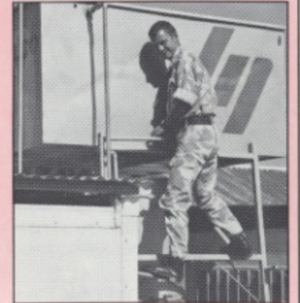
Sapper B Price puts a few finishing touches to the cold water tank.
