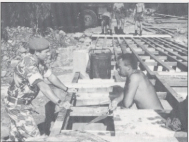
FEWO (WO1 AJ Walsh) discussing construction details with Cpl Carriage (Section Commander)
