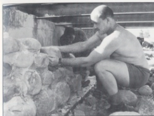
LCpl Grant assisted by Cpl Carriage placing facia to concrete abutment of bridge
