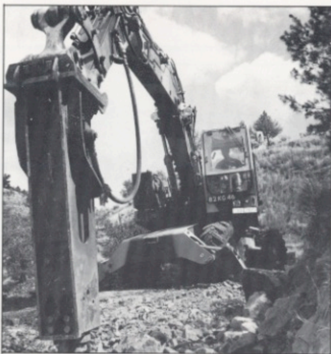
Spr Davies operating the O and K (Medium Wheeled Excavator) with hydraulic Concrete Braker attachment
