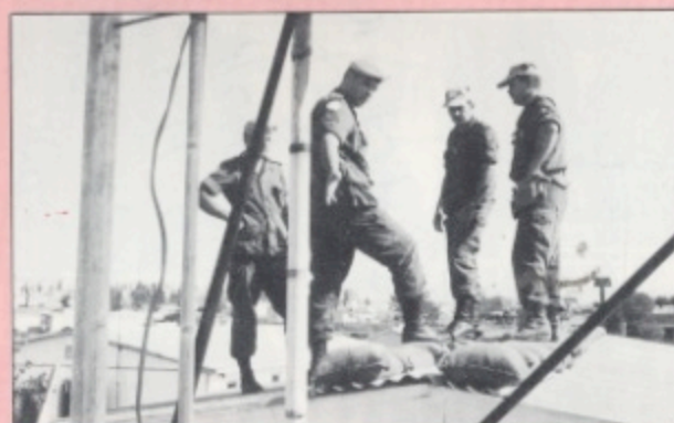
WO Lamoureux explains his plan for solving the leaking roof problem at Camp Berger.
