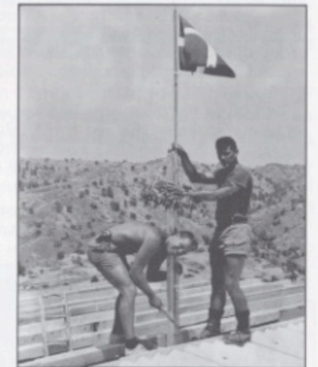
Privates 1st Class Martin Jensen (left) and Michael Hansen at D-35 on C-Coy track where the DANCON Engineers are renovating the OP.
